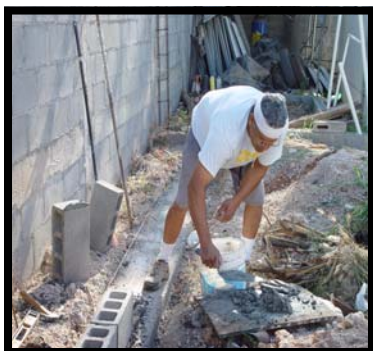
Jorge finishes footer in preparation for the cement pad on our Memorial All-Purpose building.
